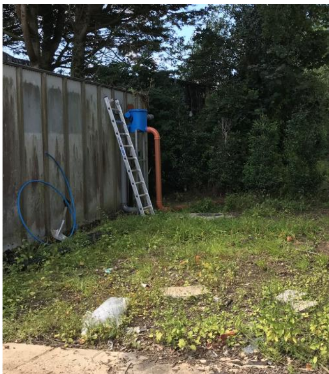
Innovative ideas implemented on site are having a positive impact on water quality further downstream. The orange pipe transports water from roof surfaces to a 216,000l tank which then feeds into the existing irrigation system on site.
