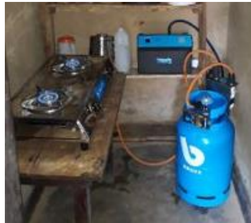
Figure 3: PAYG LPG system in a customers' home. Photo credit: T. Perros
