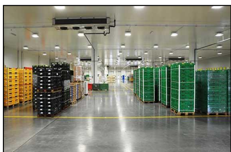
Figure 68: Modern pre-cool cold storage. 23
